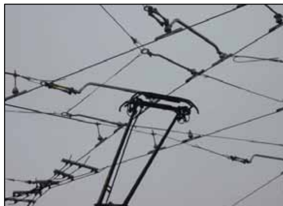
Overhead Lines on Market Street
