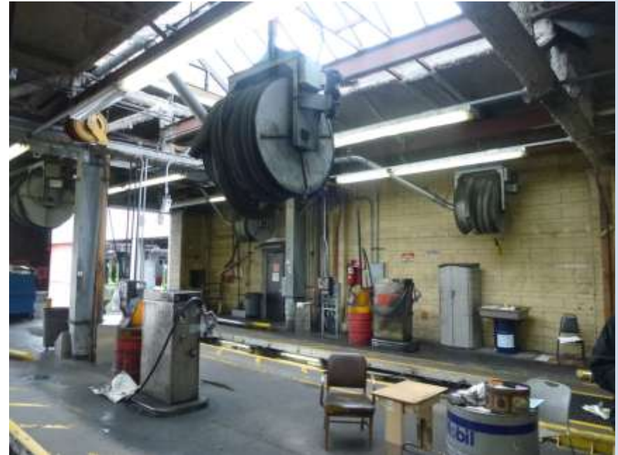
Inoperable vacuum system in fuel area at Woods.
