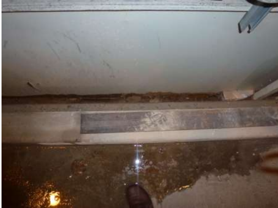
Roof leaks at Cameron Beach are causing the paint booth to rust.
