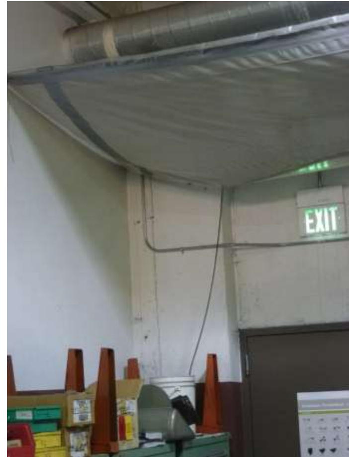
Tarp and bucket used to catch roof leaks in Parts Storage at Potrero.
