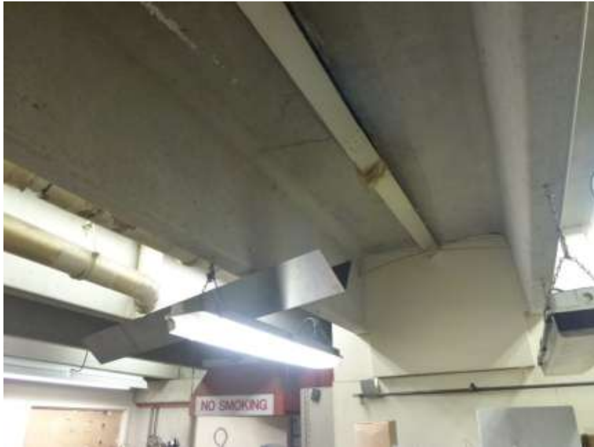
Fabricated gutters in Component Repair at Woods due to roof leaks.
