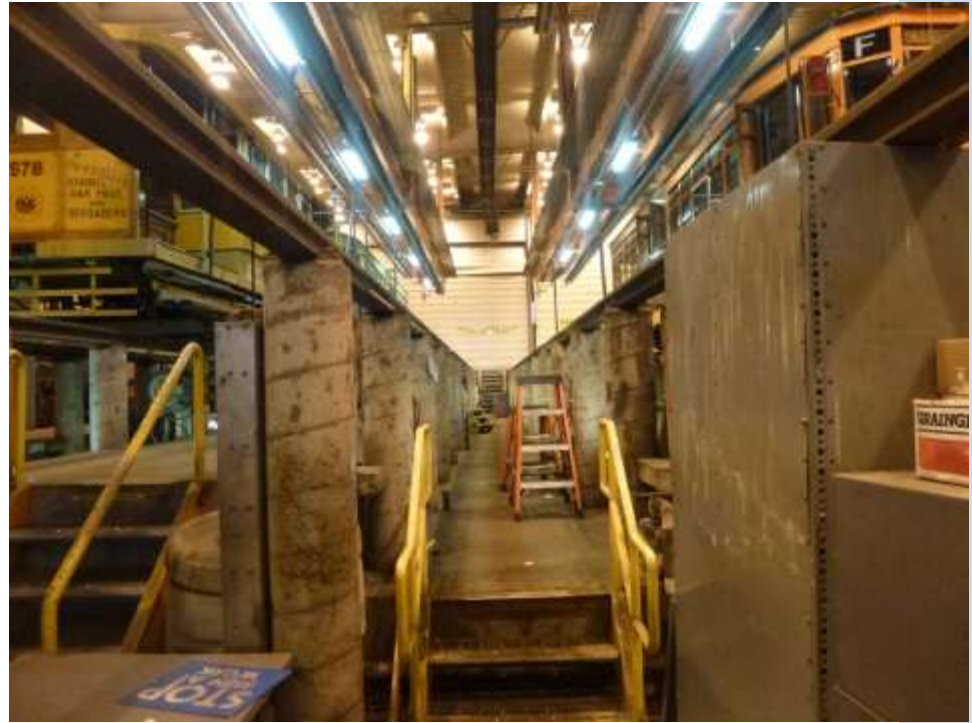
The rear doors for the repair lanes are broken and cannot be opened.
