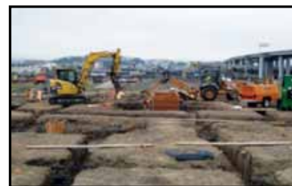
Construction of Islais Creek Motor Coach Facility is on schedule. (Photo provided by SFMTA Construction Division)
