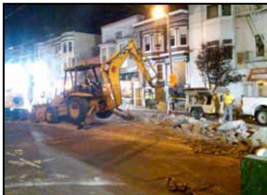
Crews worked around the clock to install a track crossover on Church Street, south of Market Street, during the Oct. 21, weekend. (Photo provided by SFMTA Construction Division)
